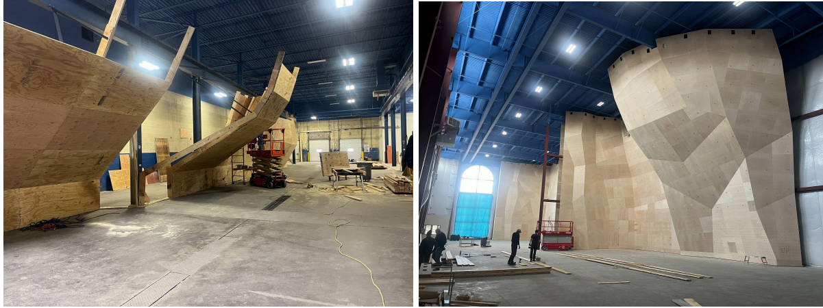
Images: Planet Rock - Grand Rapids under construction in late 2025 using untreated wood support and baltic birch plywood and direct attachment to building walls.
